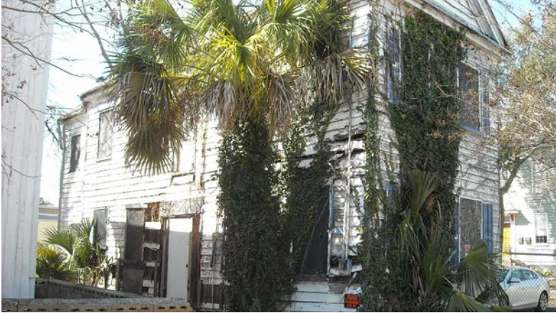
83 Nassau Street abandoned house prior to beginning renovation work. The house will be completed in 2018 with four studio apartments for men currently residing in the Mission's dormitory.
